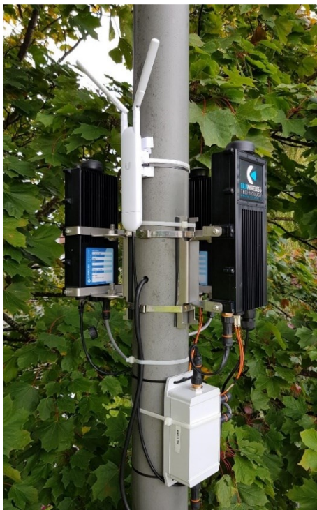
Nodes installed on a lamppost in Kensington, Liverpool
