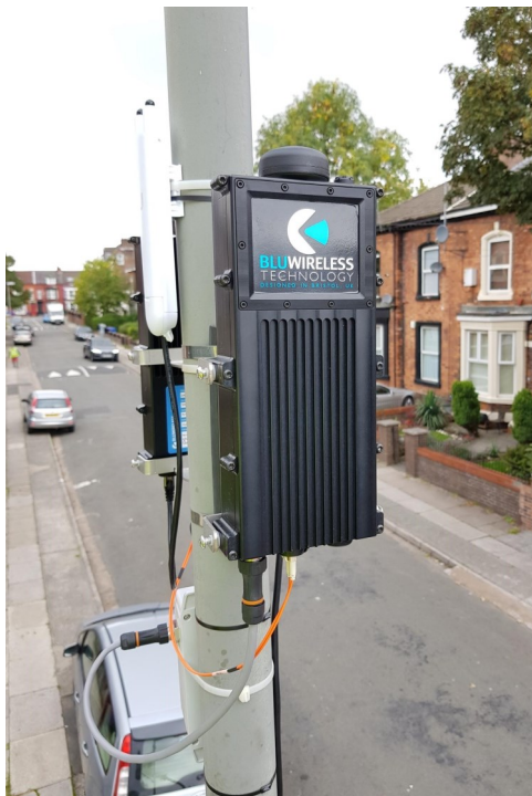
Nodes installed on a lamppost in Kensington, Liverpool
