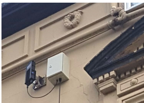
Node installed on building
